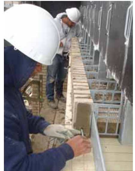
Place brick next to bracket and slide stitching rods into core holes.
